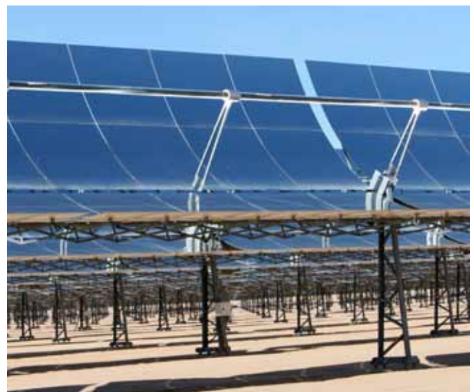
Illustration 3. Parabolic trough solar concentrators
