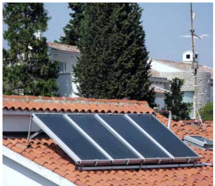
Illustration 4. Solar water heaters on a roof
